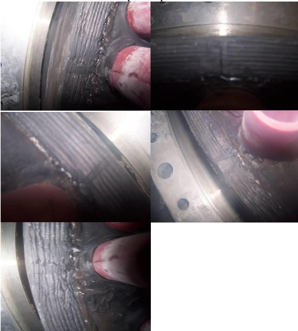
Picture 7 – 11 – Numerous poor repairs to tubesheet
