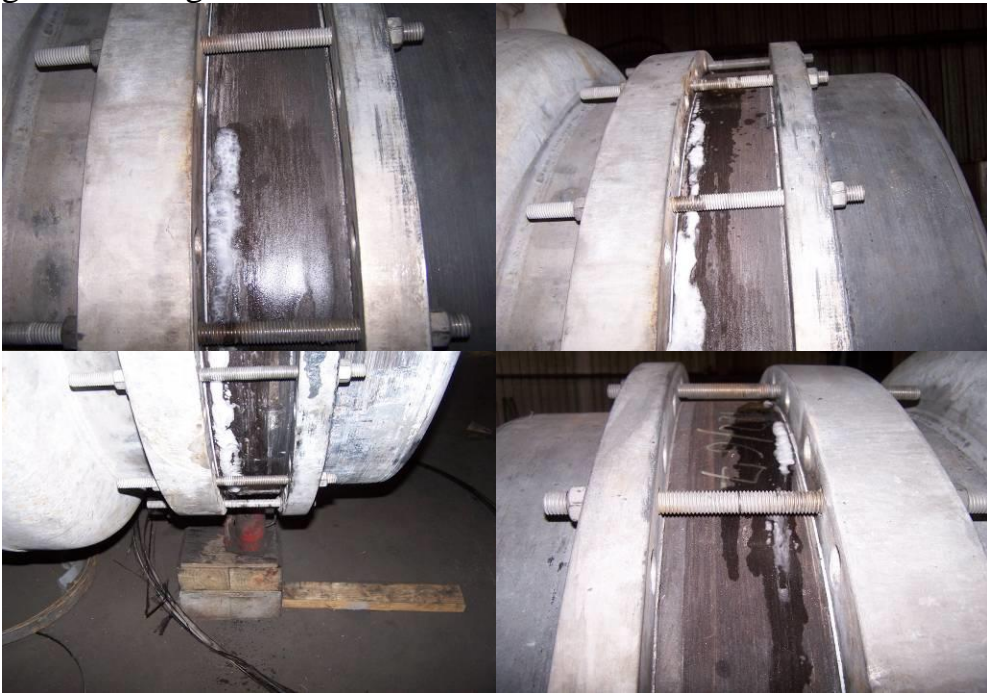
Picture 12 – 15 – Bleeding areas at gasket area found to be cause of the gasket leakages.
